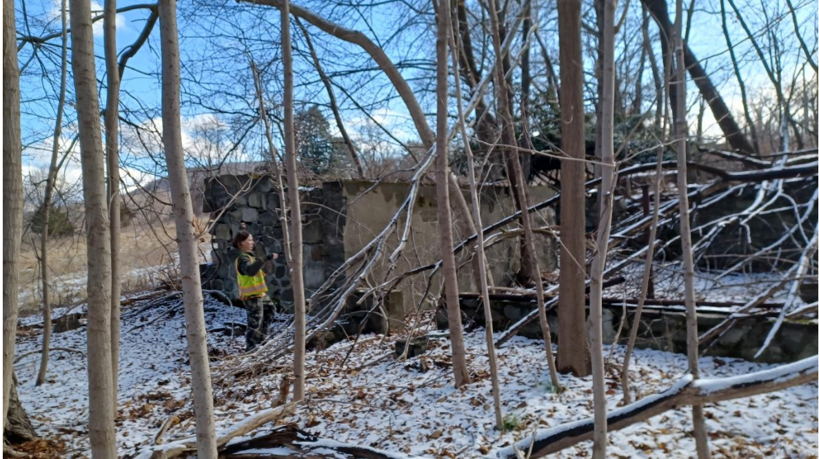
Photo 4: A foundation comprised of dry laid and mortared stone with cement facing is located to the northwest of the 1920s house. View to the northeast.
